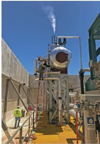
SPECIALTY WORK Rosendin Electric recently completed work on a heating and power facility for Arizona State University.
