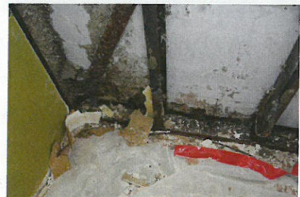
Check out the debris and damage inside this demolished wall.
