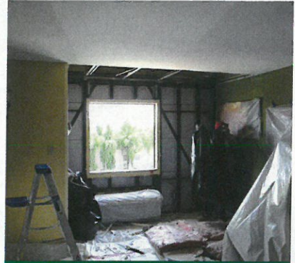
A peek inside a guest room in the midst of being dried and repaired.
