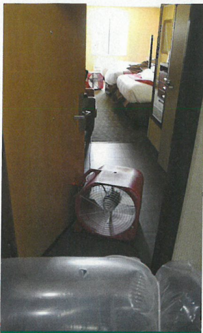
One room, two air movers. Imagine the amount of equipment needed for 165 rooms, plus larger spaces.
